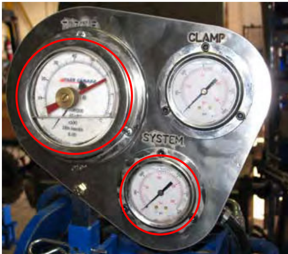
ILLUSTRATION 2.I.11: TORQUE & SYSTEM PRESSURE GAUGES ON GAUGE PANEL
